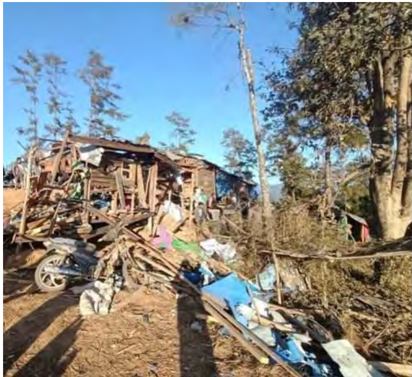
A group of young Chin villagers among the ruins of wooden builders after an airstrike, 2023. Photo Credit: CNF
